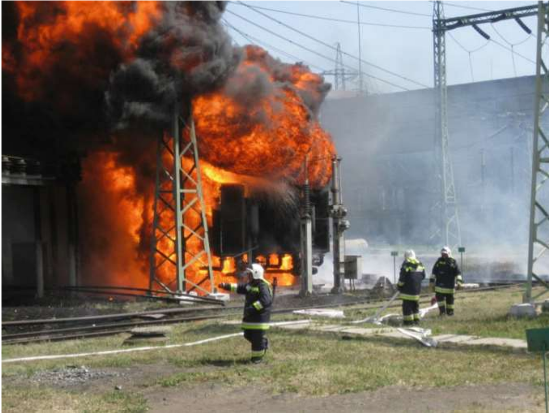
Fig. 1.7 Fire in a block transformer of a power plant, the city of Omsk, July 2011. The transformer passed a routine inspection with a complete set of preventive tests and measurements a month before the incident
