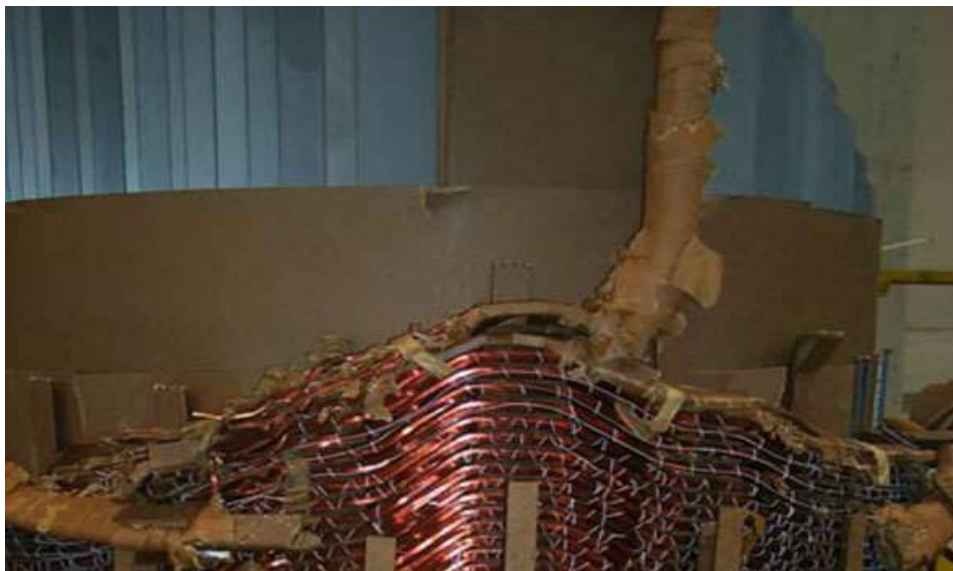
Fig. 1.14 Complex displacement of winding turns
