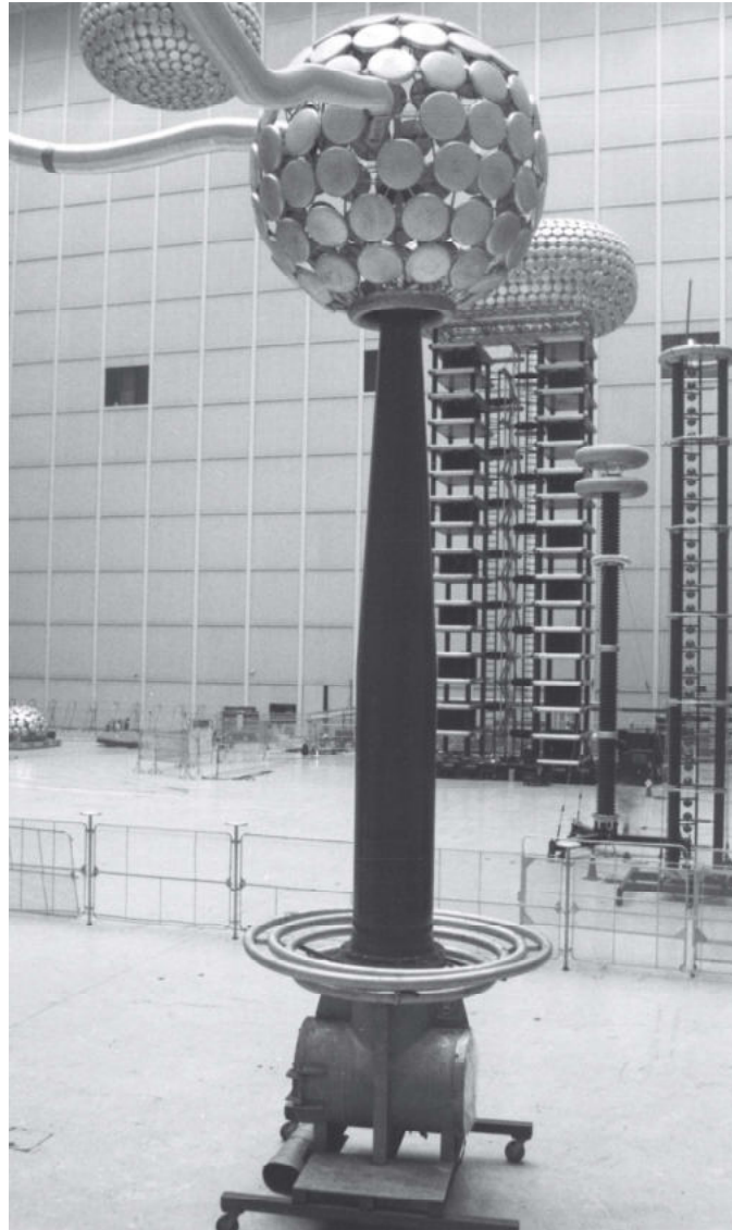
FIGURE 11.37 1 MV ac termination with fiber-glass housing at IREQ. (Photo courtesy of Hydro Québec.)
