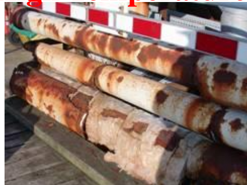
High Temperature Corrosion
