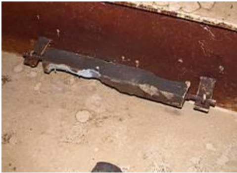
Cathodic Protection. Sacrificial Anode
