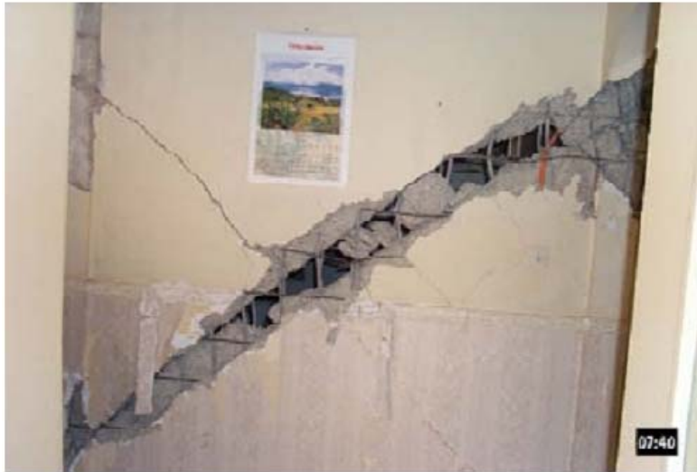
Photo 02: crack on longitudinal shear wall
