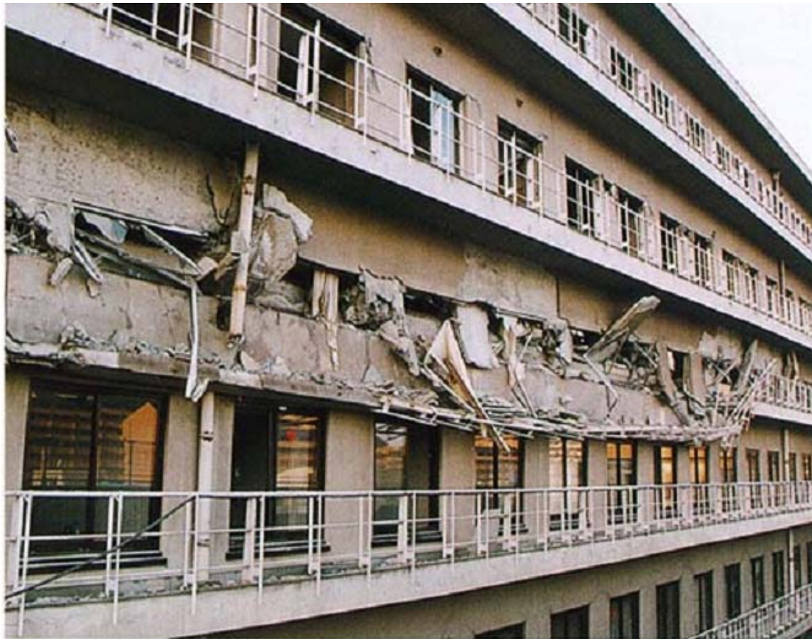
Gravity load collapse from 1995 Kobe Earthquake
